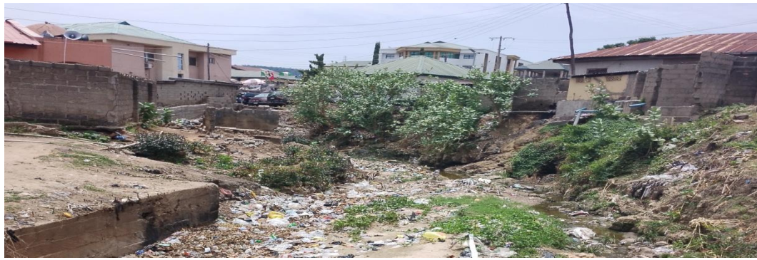
Figure 3: Poor drainage system in Ganaja Community
