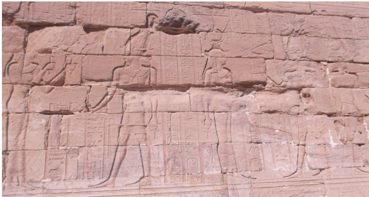
(Figure.5) Black weathering, Loss of stone material parallel to the stonesurface or profile
