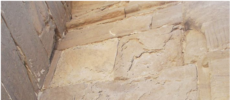
(Figure.4) Degradation of stone into thin separated layers following the beddingplanes of the rock surface
